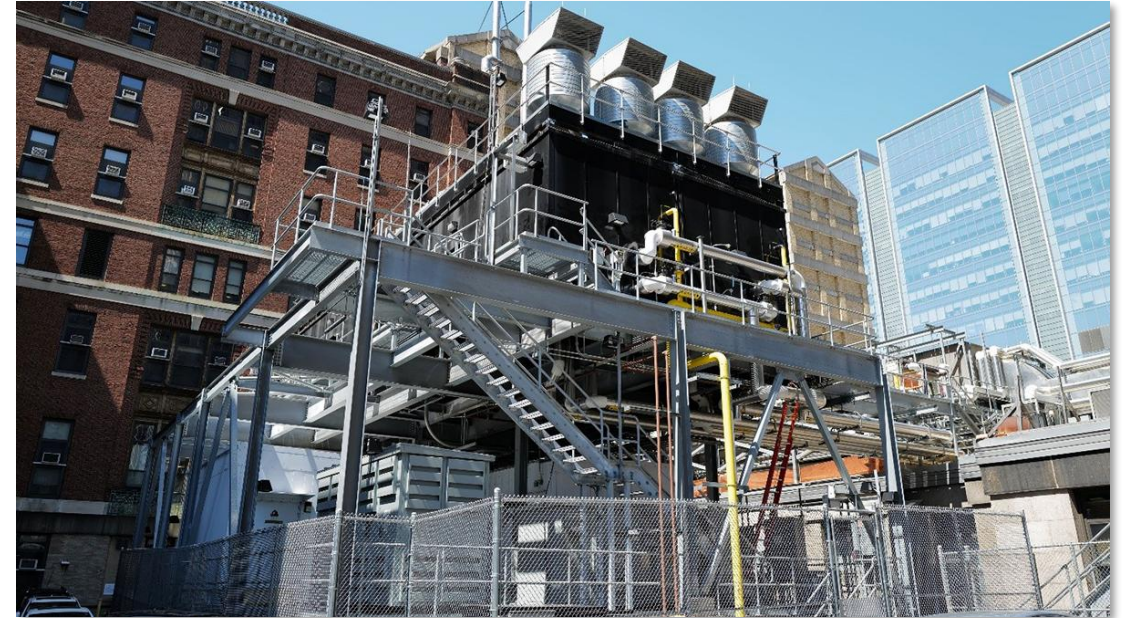
Bellevue Hospital's new cogeneration system
